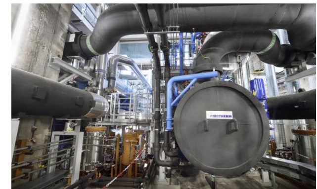
CHP cooling water heat pump (32 MW)
